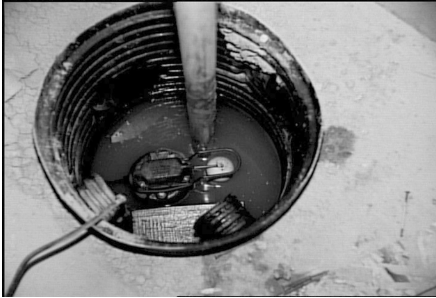
Figure R202(16) SUMP PUMP
