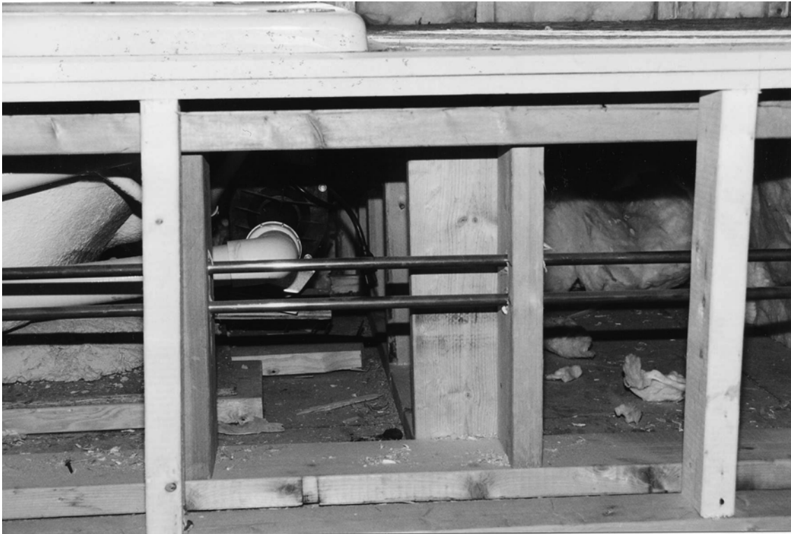
Figure P2720.1(1) NONCOMPLIANT WHIRLPOOL BATHTUB PUMP ACCESS
