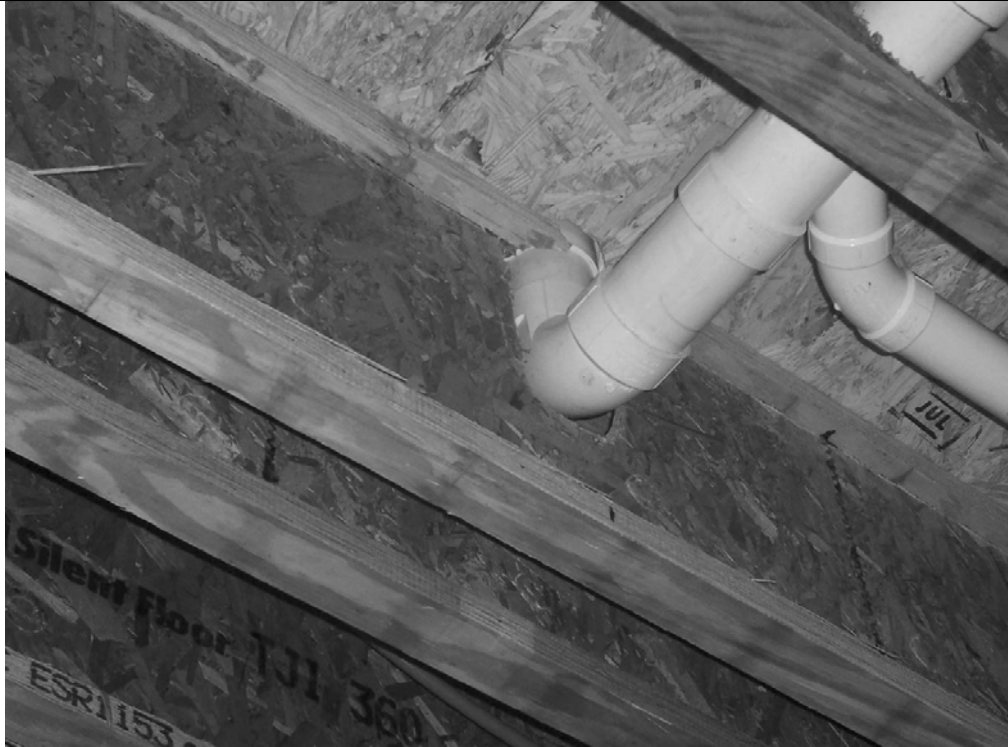
Figure P2603.2(10) VIOLATION: TOP CHORD OF I-JOIST COMPLETELY SEVERED
