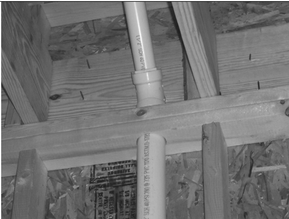
Figure P2603.2(6) VIOLATION: WALL TOP PLATE NOT REINFORCED
