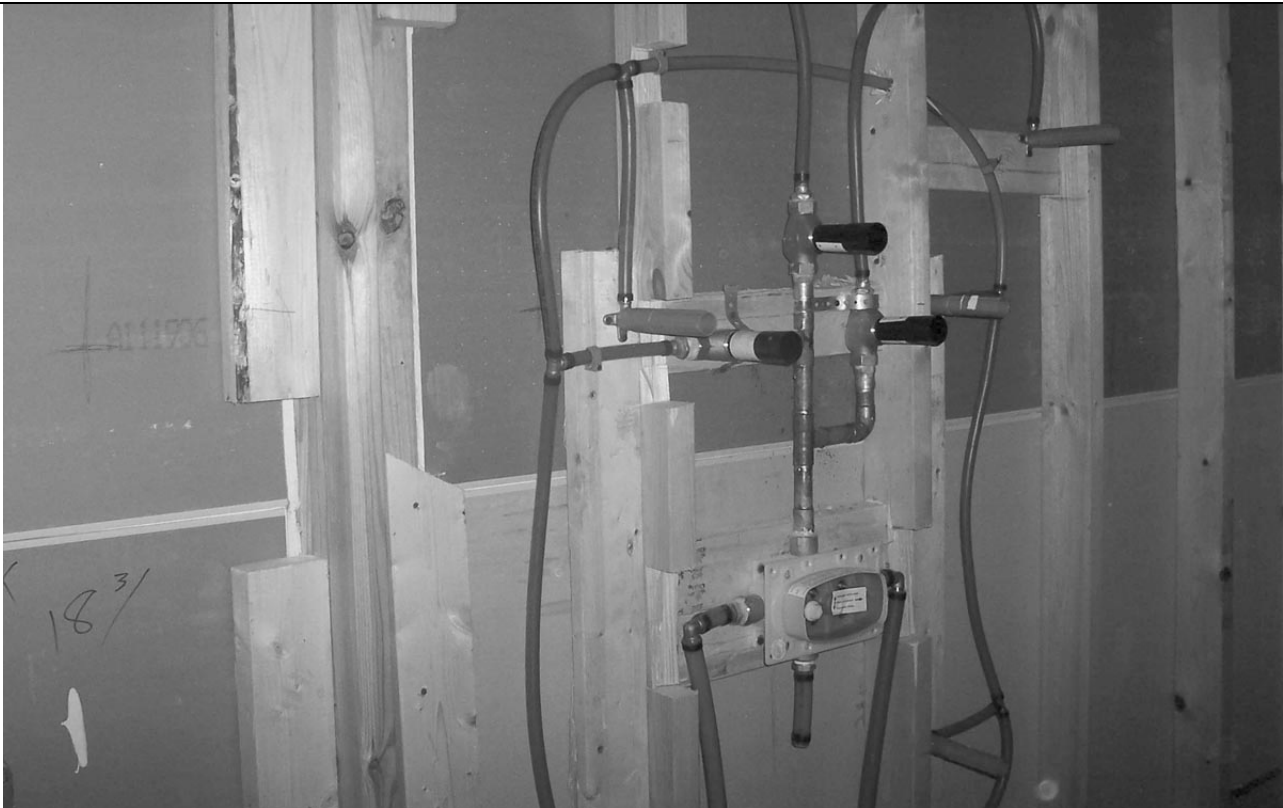
Figure P2603.2(2) VIOLATION: NOTCHES TOO DEEP IN STUDS
