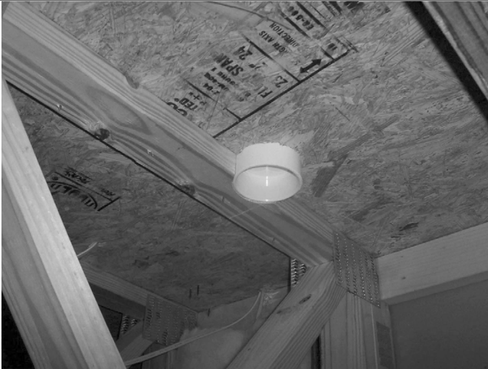
Figure P2603.2(8) VIOLATION: TOP CHORD OF TRUSS NOTCHED
