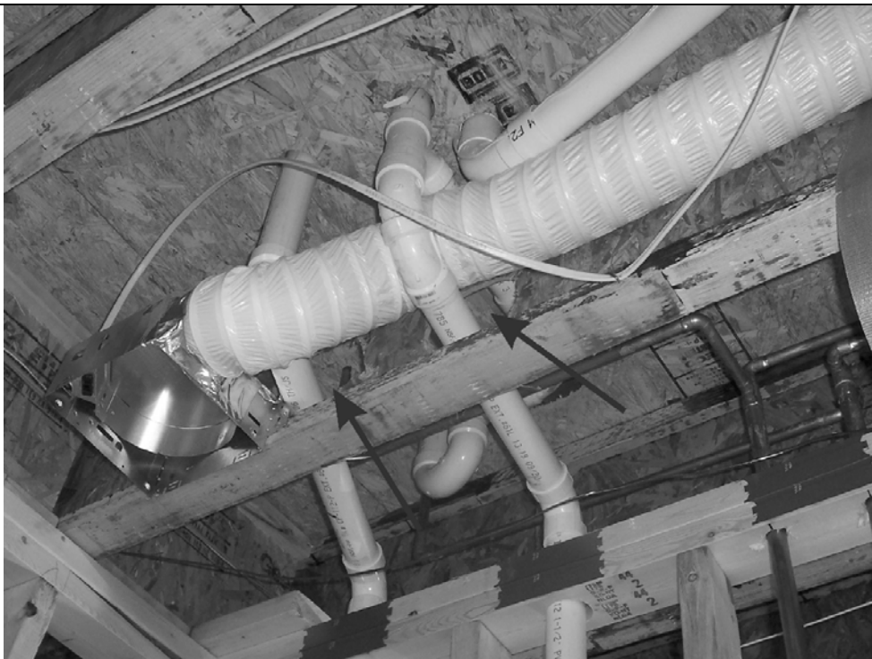
Figure P2603.2(11) VIOLATION: I-JOIST WEB HOLES IRREGULAR SHAPE, TOO LARGE, TOO CLOSE TOGETHER
