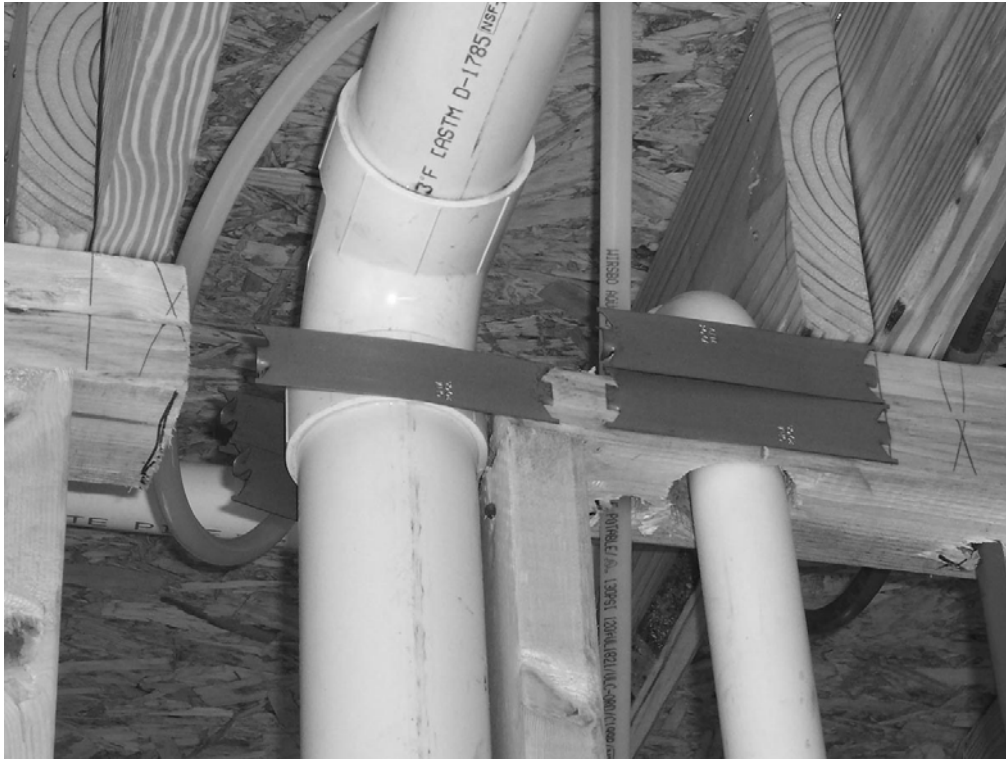
Figure P2603.2(5) VIOLATION: WALL TOP PLATE NOT REINFORCED
