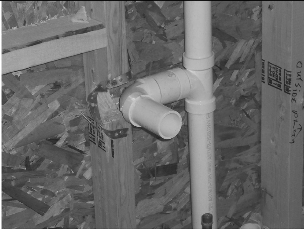
Figure P2603.2(3) VIOLATION: EXTERIOR STUD NOTCHED TOO DEEP
