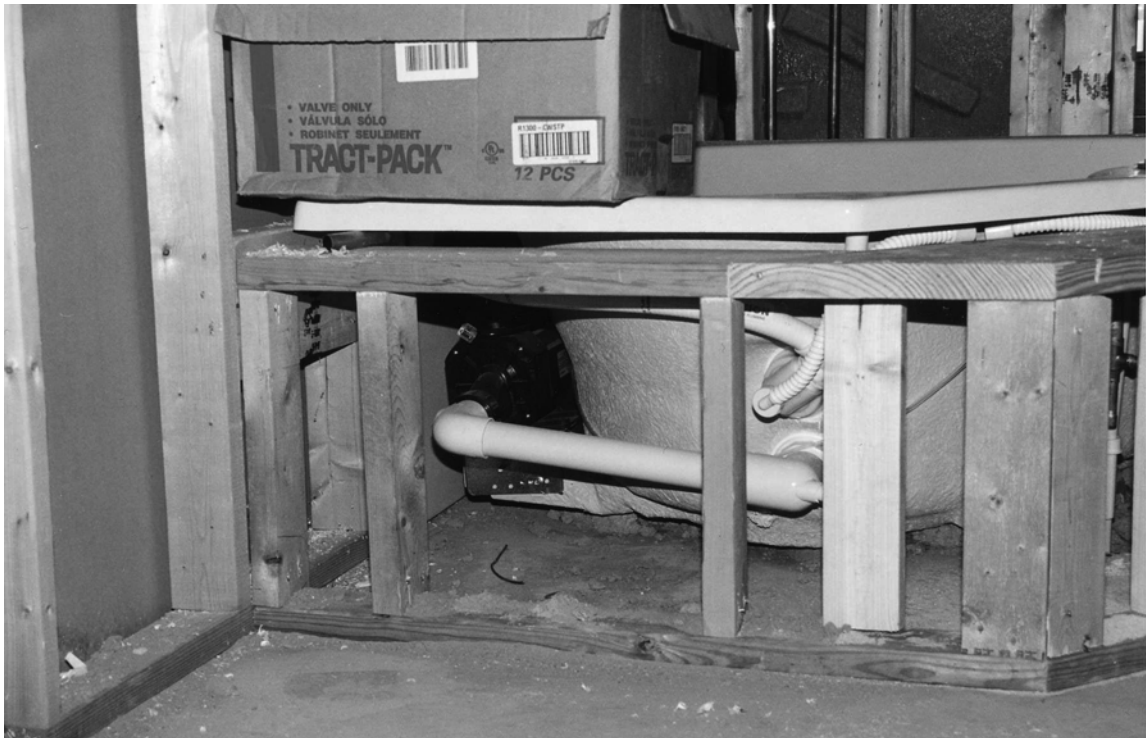
Figure P2720.1(2) NONCOMPLIANT WHIRLPOOL BATHTUB PUMP ACCESS
