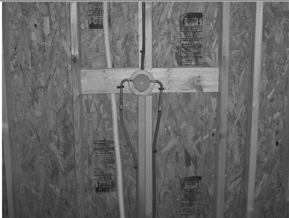
Figure P2603.2(4) VIOLATION: EXTERIOR STUD COMPLETELY SEVERED
