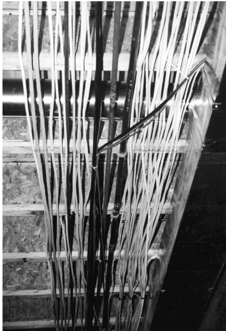
Figure E3802.4 PROHIBITED INSTALLATION OF TYPE MM CABLE ACROSS THE BOTTOM OF FLOOR JOISTS
