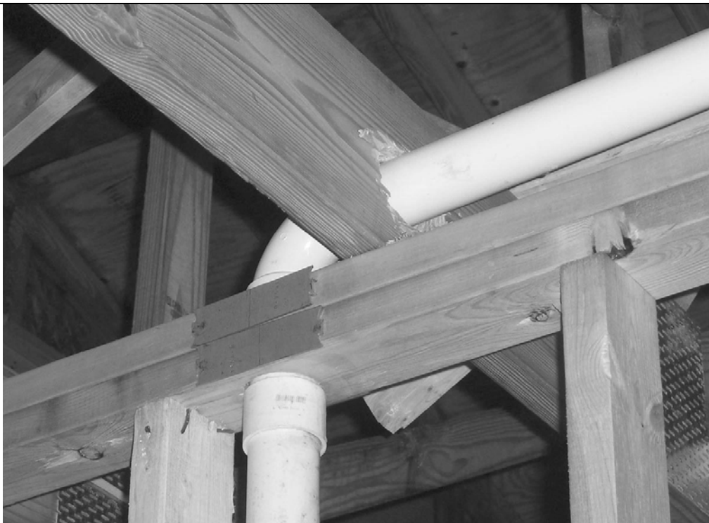
Figure P2603.2(9) VIOLATION: HOLE IN BOTTOM CHORD OF ROOF TRUSS
